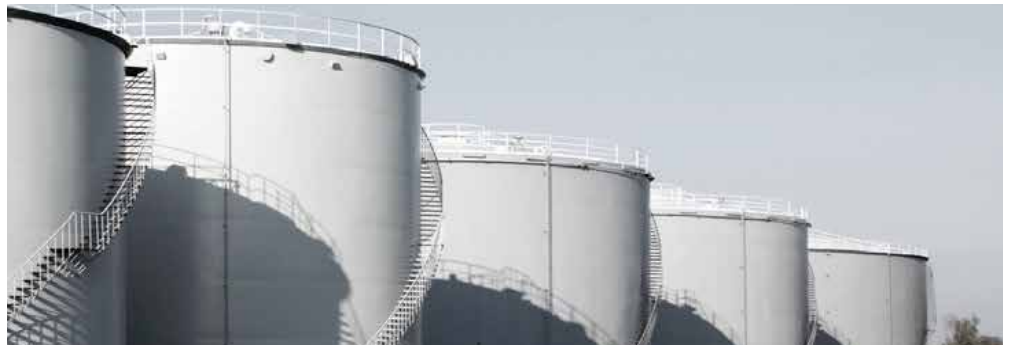
Industrial water tanks
