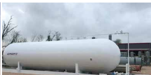
Fuel and gas tanks
