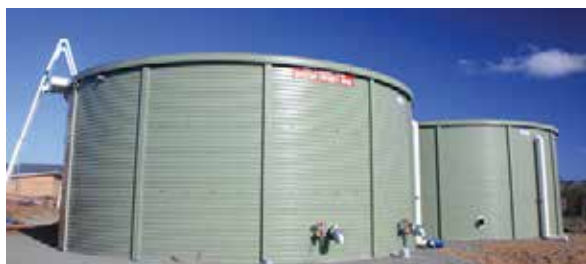
Residential water tanks
