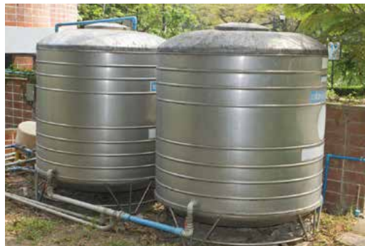
Domestic water tanks
